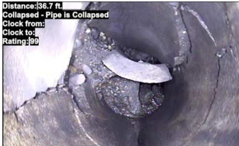
Screenshot from assessment video showing full pipe collapse
